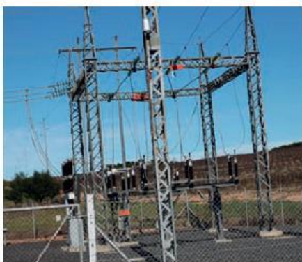
Steel electricity pylons
